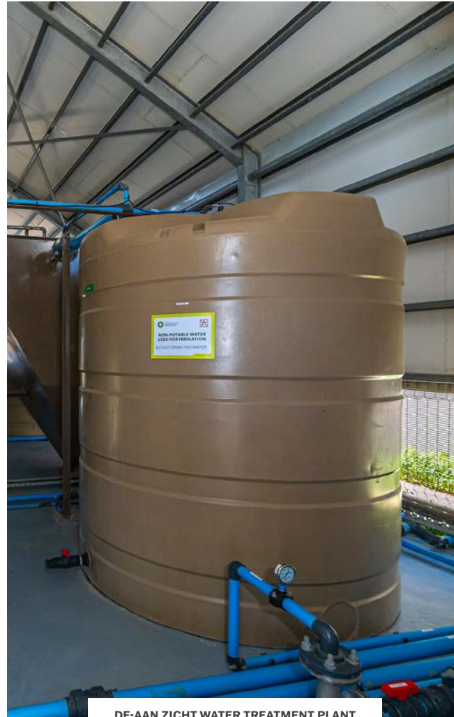
DE-AAN ZICHT WATER TREATMENT PLANT
